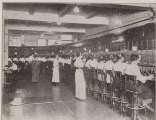
A MODERN BELL-TELEPHONE SWITCHBOARD
